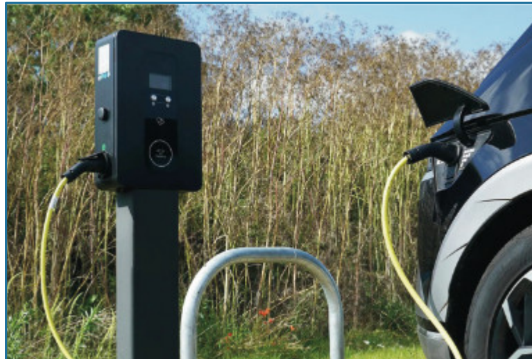
Fig.66 Floor mounted EV charging point
