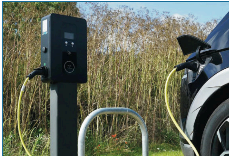
Fig.66 Floor mounted EV charging point
